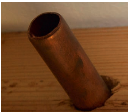
Open-ended copper gas pipe which is classified as immediately dangerous (ID) and RIDDOR reportable to the HSE
