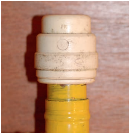
Plastic push-fit cap which is not fit for purpose on gas installations and is RIDDOR reportable
