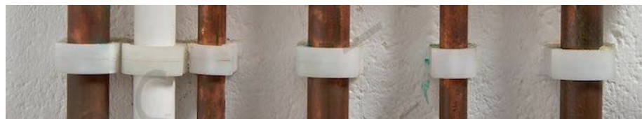
Pipework should be properly and effectively supported and installed to avoid any undue risk of damage
