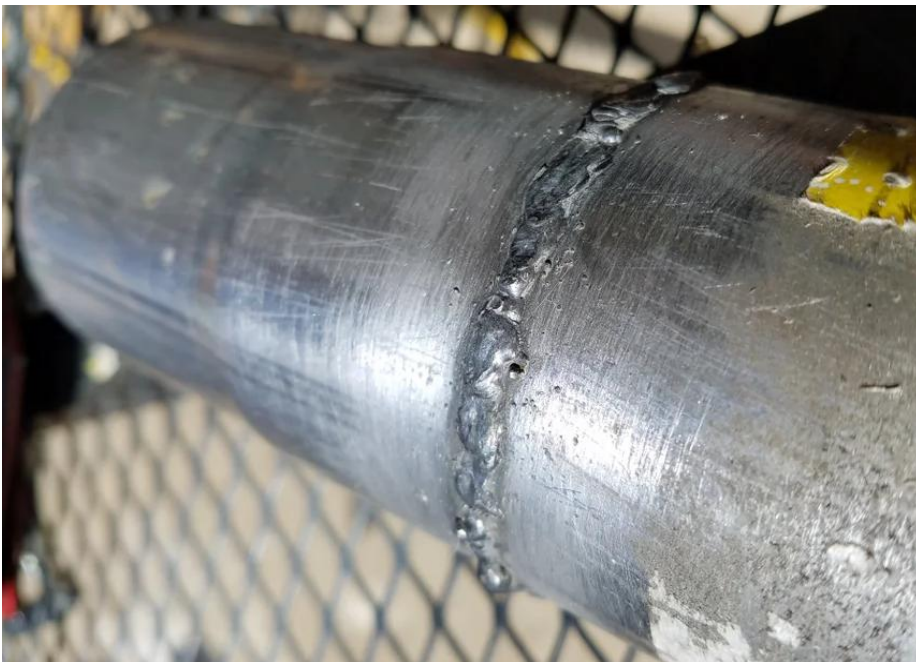
Photograph 2: Photographic evidence shows the welded joint between the exhaust pipe and extender, showing the level of quality finish with bubbles and a difference in weld thickness throughout the join.
