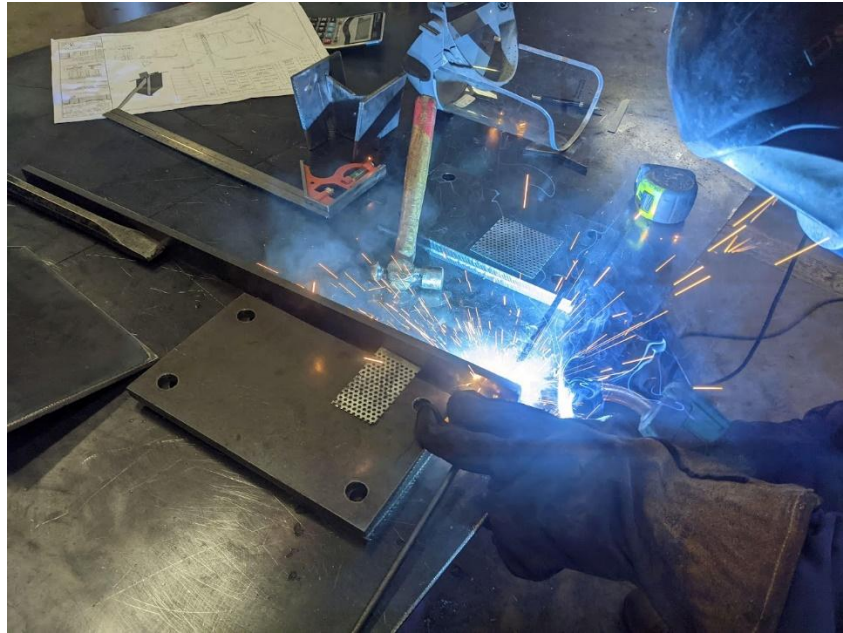
Photograph 16 – showing application of tack welding, note the damage to the component.
