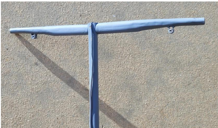
Photograph 12 shows the insulation fitted to the cable fixings.
