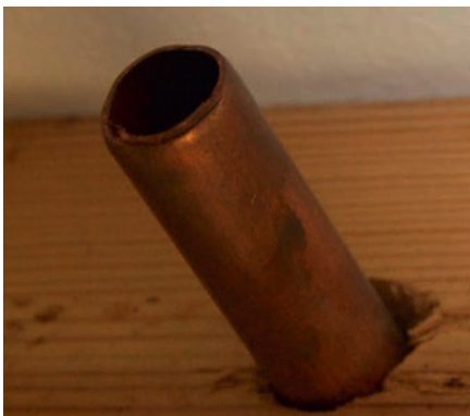
Open-ended copper gas pipe which is classified as immediately dangerous (ID) and RIDDOR reportable to the HSE
