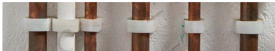
Pipework should be properly and effectively supported and installed to avoid any undue risk of damage
